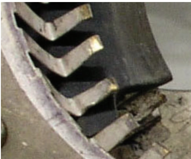
Figure 7 Bent and broken finger stock. Finger stock may become damaged due to effects of overheating or mishandling. Any broken finger stock must be repaired or replaced immediately to ensure long tube life.
